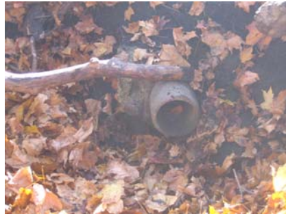
Figure 2. The cement pipe above is the outlet at the head of Ravine Z, and about 8 inches of cement is visible to the left of the pipe which is only visible after headward erosion.
